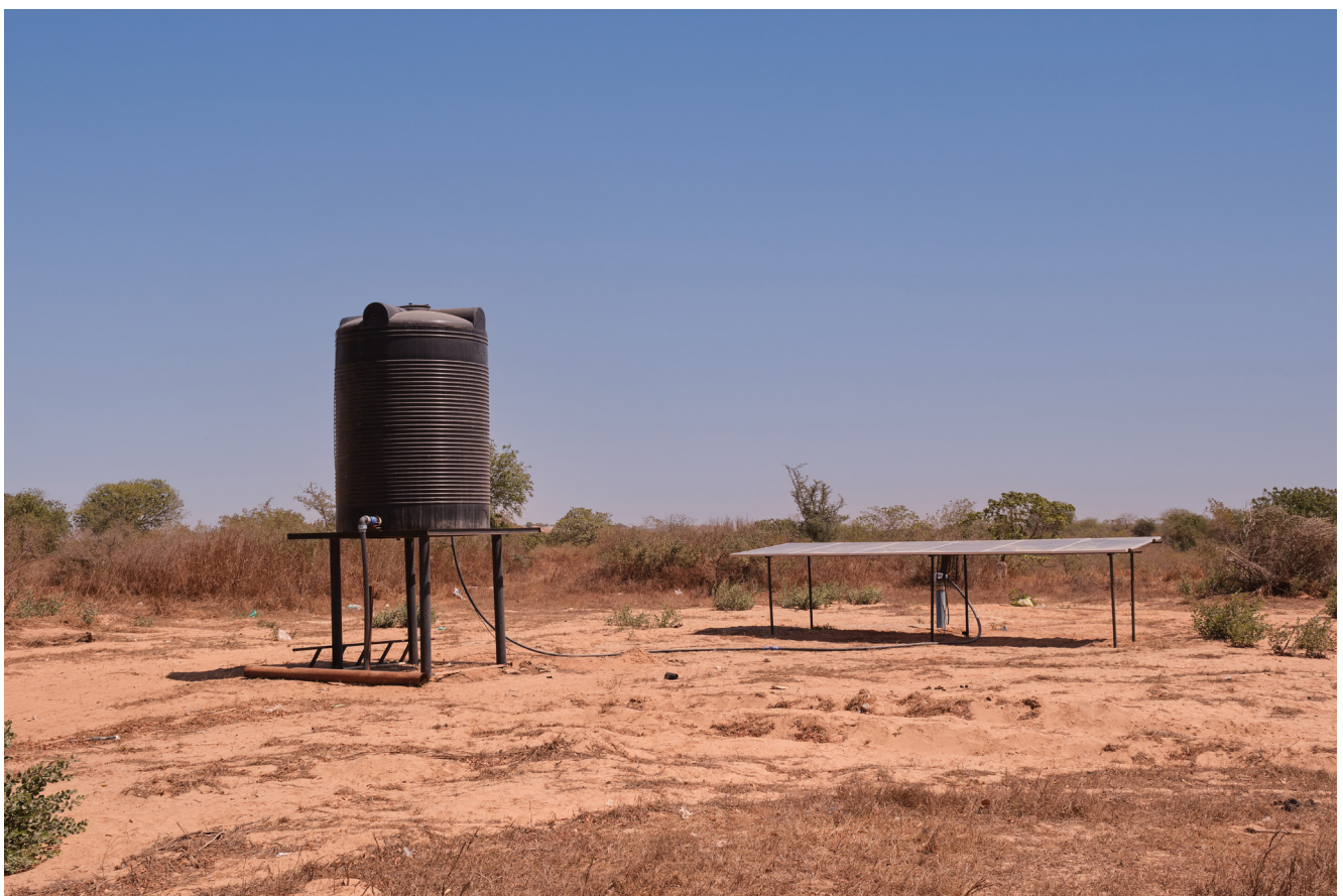
A network of borewells established to supply drinking water to the local communities in Senegal
