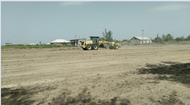
Before: Levelling work underway on a football field at a local school in Uzbekistan After: Students enjoying a game of football on the newly levelled school ground
