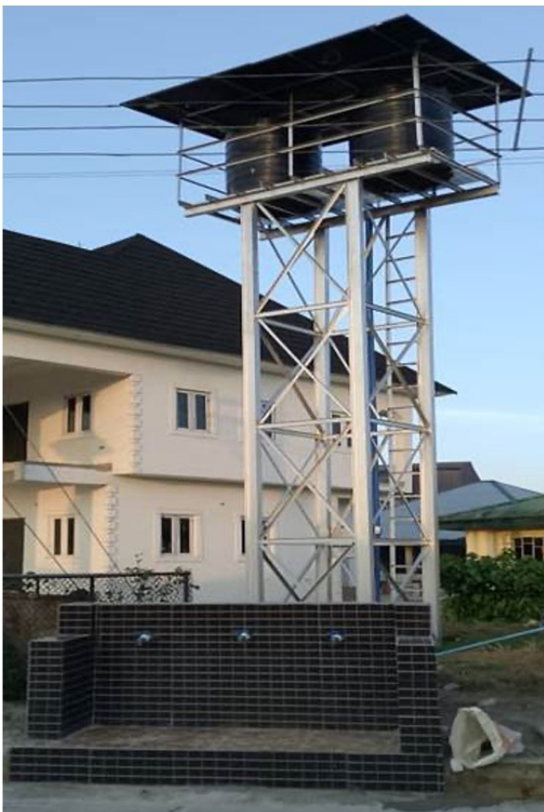
Solar powered water borehole installed in the Njuru community, Nigeria
